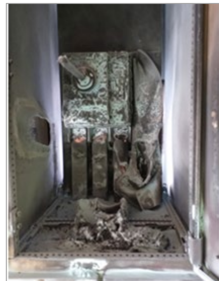
Figure 10-2: Electric arc damage in 415v switch panel - tools melted at front, hole where the left-hand panel vapourised Source: RMS.
