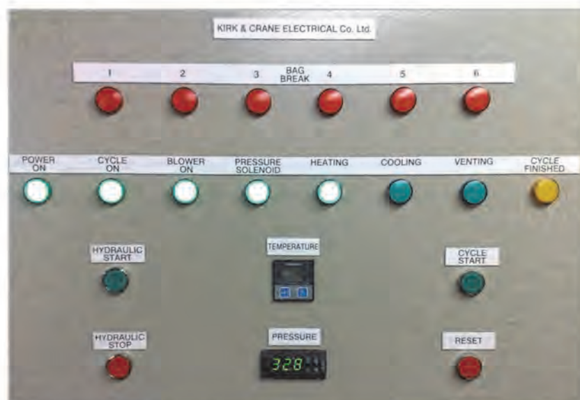
Figure 7-3: Control panel – clear layout and markings.
