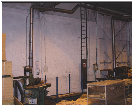
Figure 8-4: Length of ducting with curves. Source: RMS.
