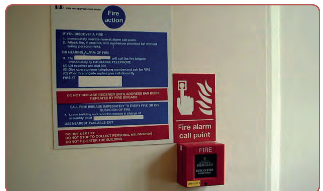
Figure 2-6-49: Alarm point identified and well located. Source: RMS.
