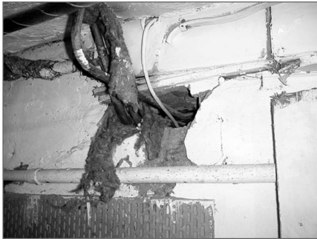
Figure 4-1: Opening not fire stopped.
