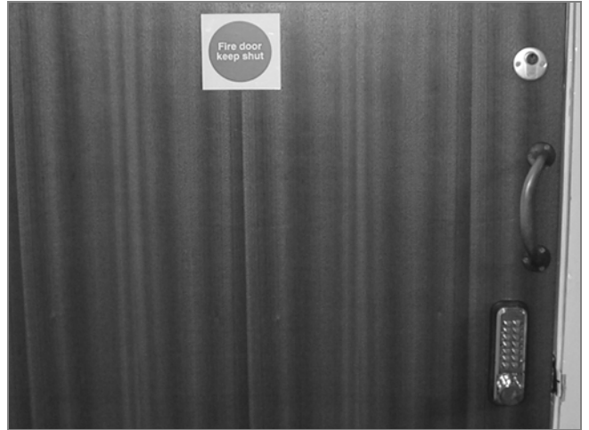
Figure 3-16: Access control, internal security. Source: ACT.
