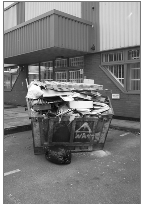
Figure 3-17: Poor siting of skip. Source: FST.
